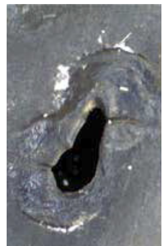
Sun damage to the dripperline
